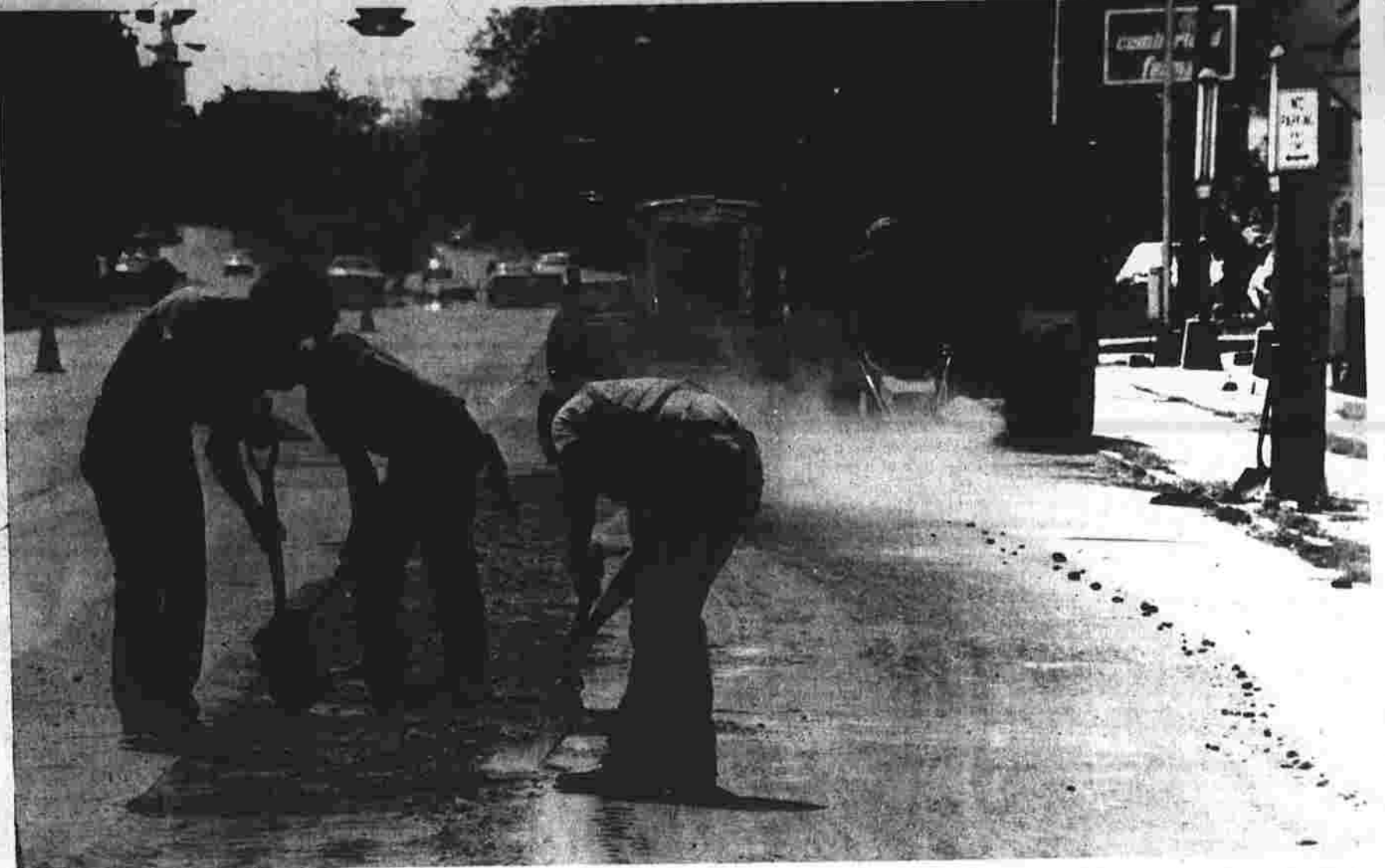
Manchester is getting scarred and patched up with construction in progress all over. Workers here at East Center Street near Lenox Street are patching a spot where there was an excavation. At right a workman sweeps up with a motorized sweeper. (Herald photo by Pinto)
